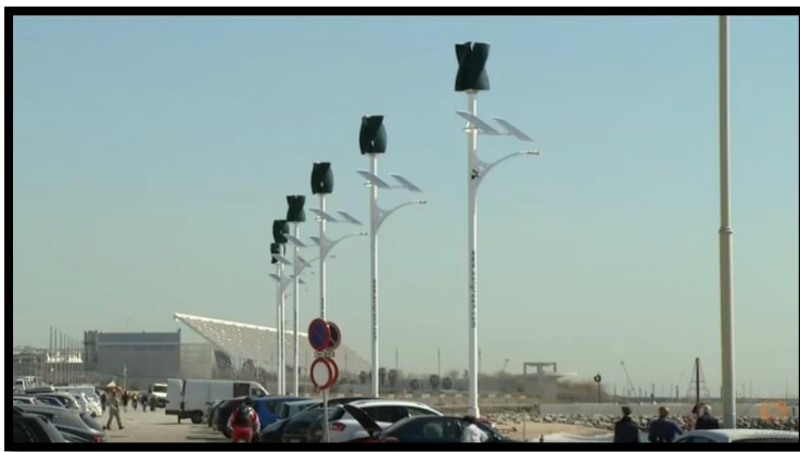
Photo 3: Street light powered by solar panels and small scale turbines in Barcelona northern beach. Source: Reuters
